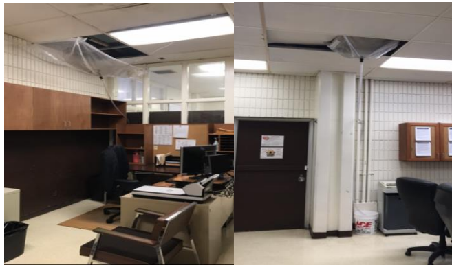
(Accreditation Section office showing plastic canopies and tubes used to catch dripping water in office work areas)
