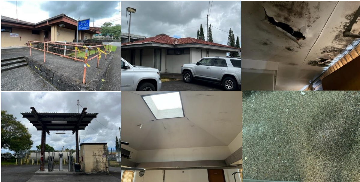
Kea'au Station and old courthouse in deteriorating condition with water damage
