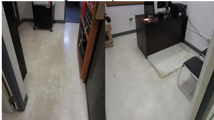
CONDITION OF POLICE STATION FLOOR (INTERIOR)
